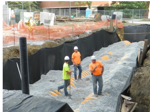
Polyethylene retention cells installed under the roadway help slow the release of surface runoff to local waterways.
